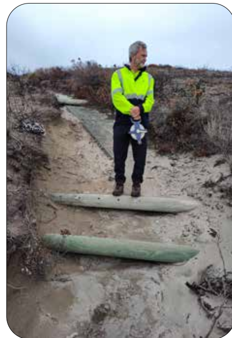
An eroded section in need of repair.
