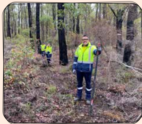
Newmont Boddington (NB) staff joined SV's for a day constructing the trail.
