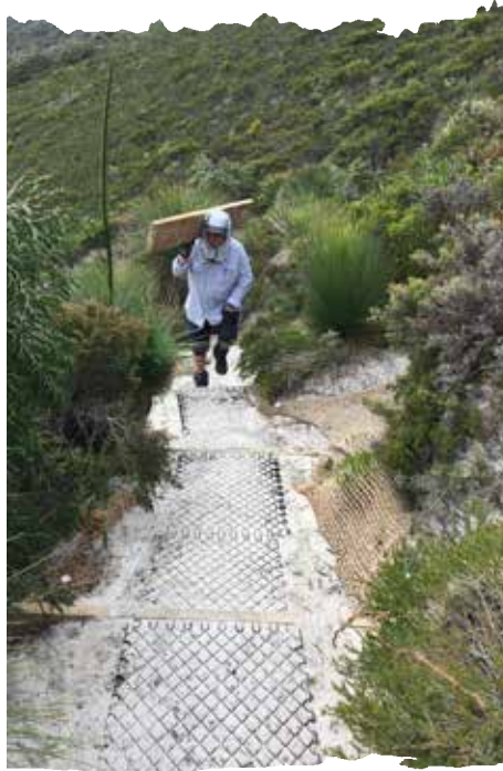
Many timber sleepers had to be moved from the bottom to the top of the hill before work could start.
