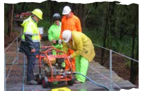
That rascally high pressure pump resisted attempts to get it running until the trouble was diagnosed and repaired.
