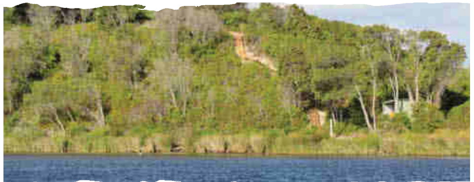
Box steps were built up the eroded slope from Irwin Inlet south side.
