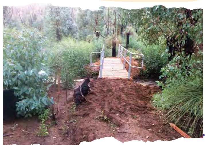
New bridge over Bell Brook, constructed with the help of Support Volunteers Ben Blomfield and Wes Fokkema.
