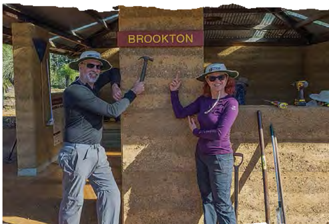
BTF volunteers, Andy and Michelle Nelson install the campsite sign. The couple are heading off on an end-to-end soon and are pleased to see all the campsites re-opening.
