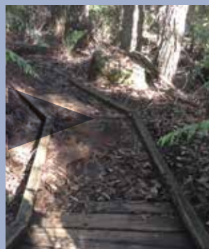
Next visit - clogged again!
