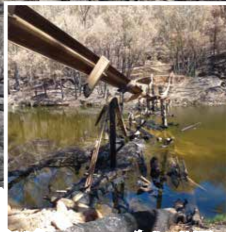
Southampton Road Bridge has been destroyed
