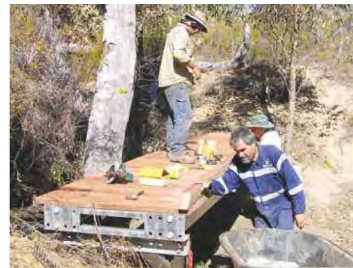
New bridge in place. Scott, David, Jim fitting side kick-boards. New trails to each end of bridge not yet complete.
