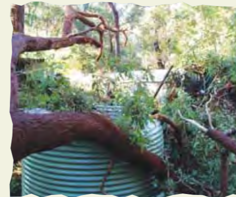
Massive branches engulfed the water tank and shelter
