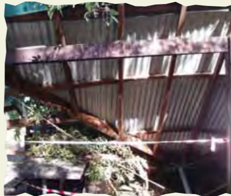
Blown down by the winter storms, a giant Tingle tree caused major damage to Giants campsite.
